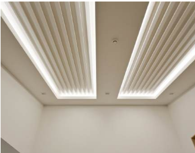
Fall Ceiling With LED Light
